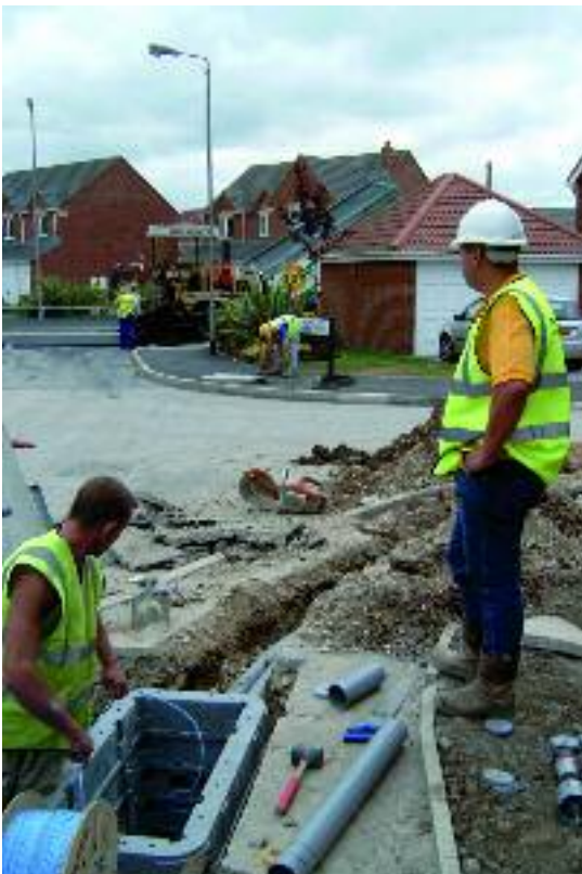
Salmor chambers on a private development site
